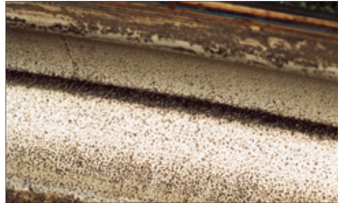
Photo 7-9-1 Part: Outer ring of a slewing bearing Symptom: Pitting occurs on the raceway surface Cause: Rust at bottoms of indentations
